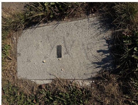
Figure 5: image showing one of the Quickline fibre chambers along the lane
